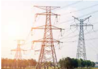
Live line installation on BOOM basis 138 kV line MTCIL (JV with MSETCL)
