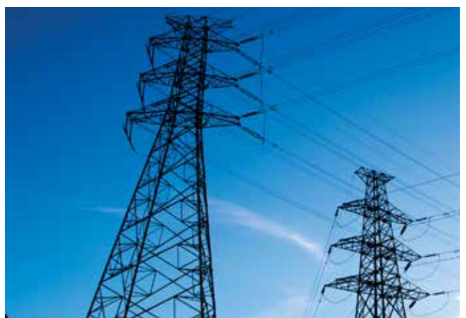
MULTIPLE LINE CROSSING - Multiple line crossing in Orissa, India (132 kV)
