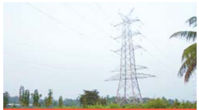
Multi circuit towers
